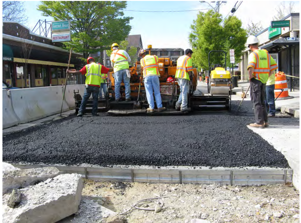
Crews from the Combined Sewer Overflow Program being run by the Narragansett Bay Commission began repaving Hope Street during April in 500-foot sections such as this one in front of Citizens Bank. According to the contract schedule of the John Rocchio Corp., the work is to be completed by Aug. 15.
