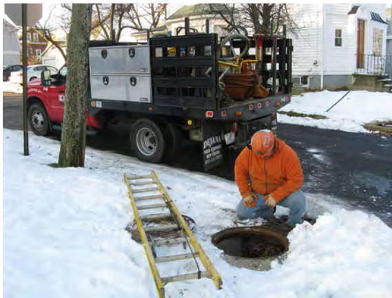
Utility work is continuing on side streets through the winter as allowed by the weather.
